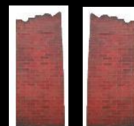
Brick Wall Flats (weathered)
